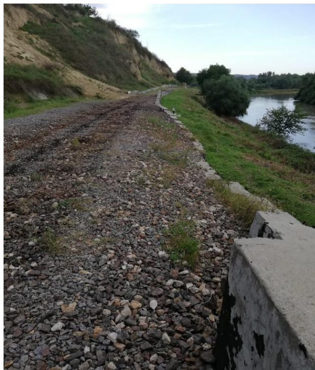
Figure 4. Displacement of the retaining wall due to the landslide process.
