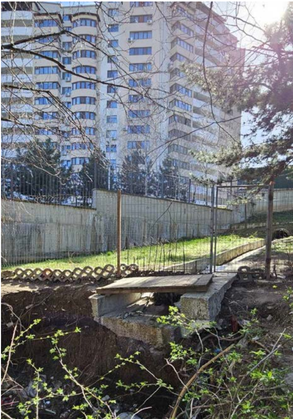
Figure 1. The damaged drainage ditch, which became the cause of the gully formation.
