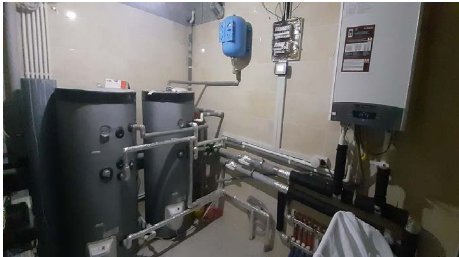
Figure 5. Gas boiler and hot water boilers.
