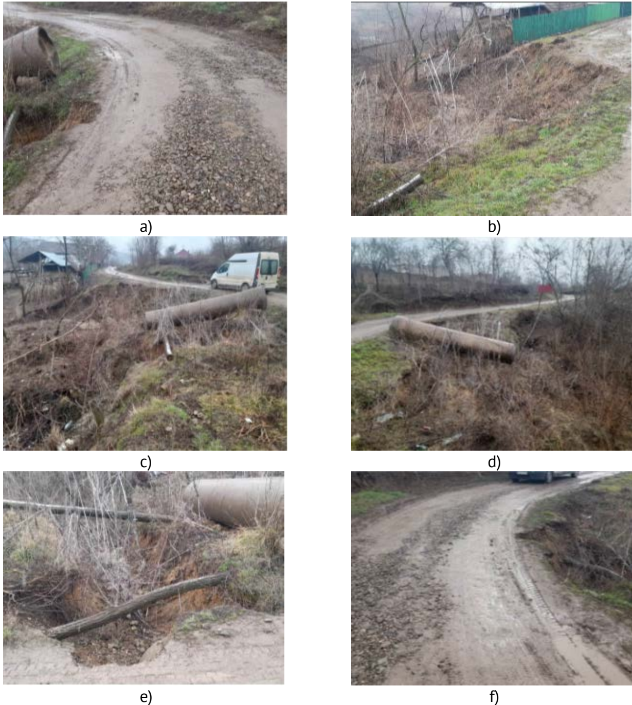
Figure 1. The analyzed landslide.
