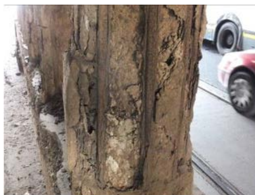
Figure 8. Degradations of the pillar support [6].
